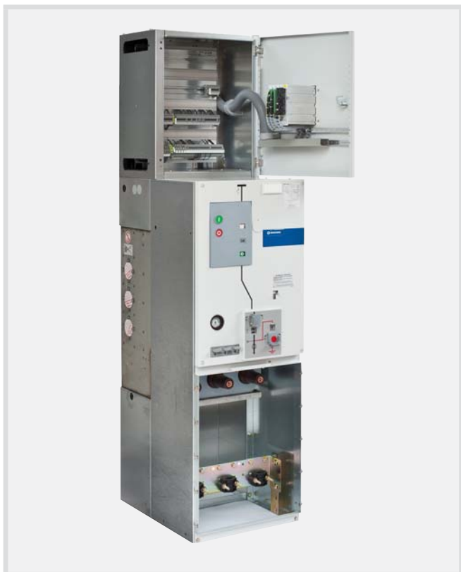
-1LSV-/5/ with opened cable front cover and relay cabinet cover
