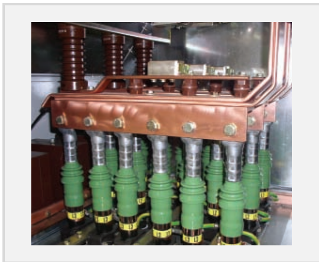
Panel type AMC9-12/2500-2500/31-L cable connection area with 6x1x500mm 2 per phase and capacitive insulators
